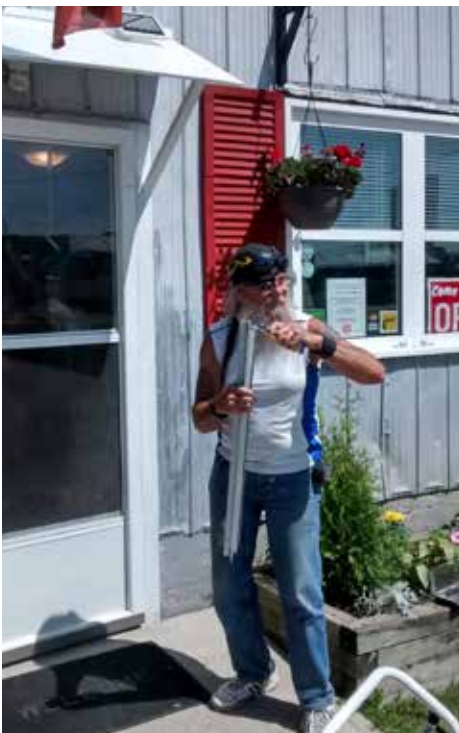
Above: Jack Jodrell, volunteer extraordinaire, puts finishing touches on new door and awning he has installed.!
